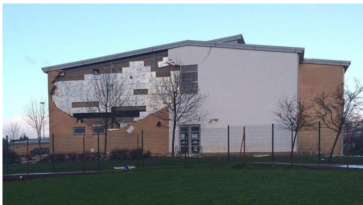
The south gable of Oxfangs School in Edinburgh after the January 2016 collapse. Picture: STV
